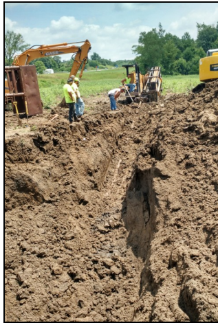
Lawson Construction crews boring under the Chariton River prior to pulling a casing and replacement water line to replace a broken main in July, 2015.
